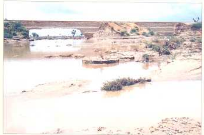
Fig. 4. Breaching of the Jaswant Sagar dam on the Luni.
